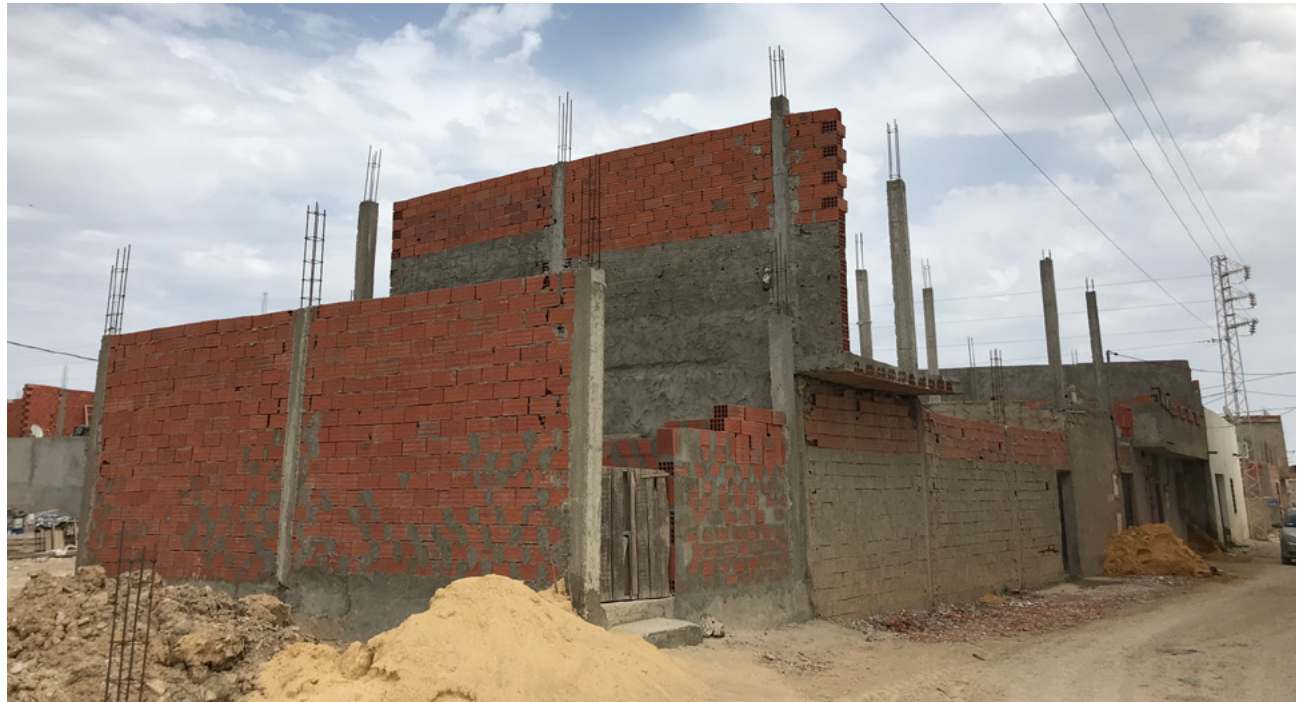
Buildings under construction in a Tunis neighborhood targeted for ARRU's upgrading program. Red bricks often signify that citizens are self-constructing, either expanding upon buildings in informal areas or making improvements to existing homes. ARRU's programs provide basic service connections and funds for improvements to toilets, bathtubs, and sinks, but not the construction of homes.
