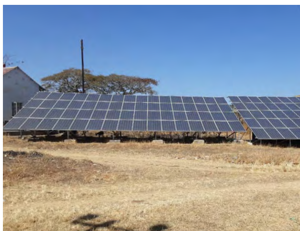
Figure 5. Installed solar panels at Makumbe Mission Hospital (Photo: CFA)
