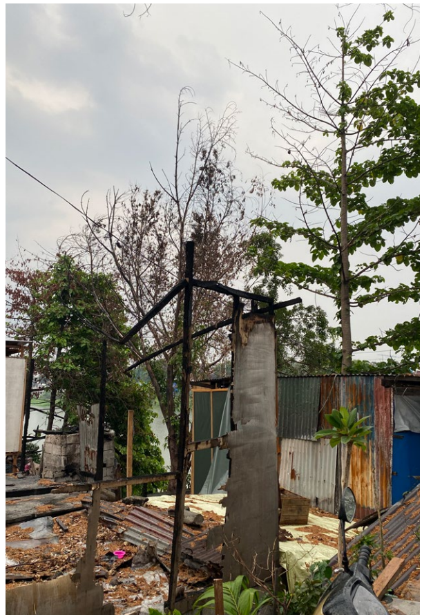
Figure 2. Informal settlement structure damaged by fire
